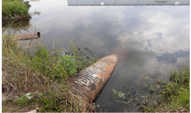
Joints fell into creek
